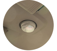
4. LED interior lighting
