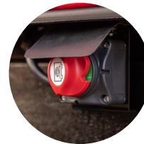
2. Battery shut-off switch
